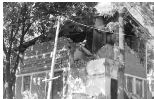
Figure 6.1 : A Damaged Building Due to an Earthquake
